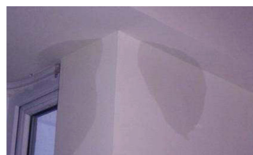
Inspect water leakage in property
